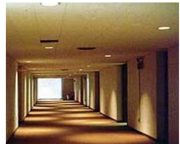
Downlights can cast confusing patterns on floors if spaced too far apart from each other or used improperly.
